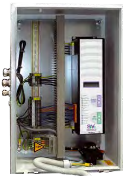
Control unit in switching box
